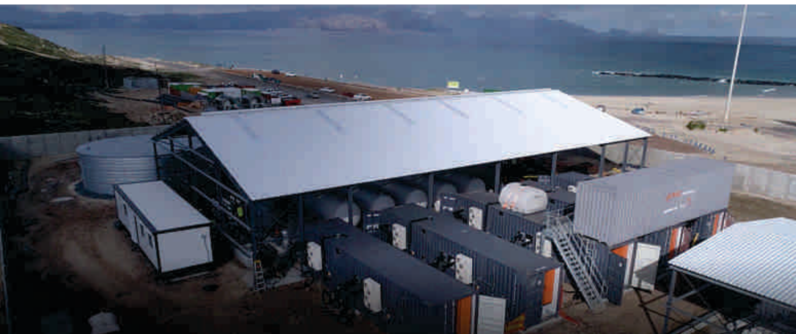
Photo: Strandfontein Seawater Desalination Plant, Cape Town, South Africa
