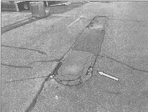
View of typical cracking and potholes in the asphalt pavements located on the north portion of the Site.
