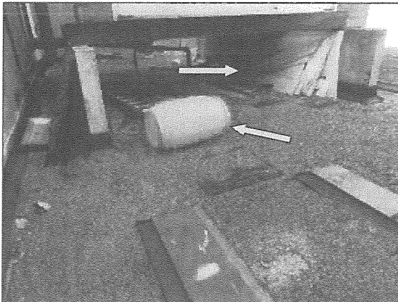
View of typical debris noted atop the BUR system within the vicinity of the cooling tower.
