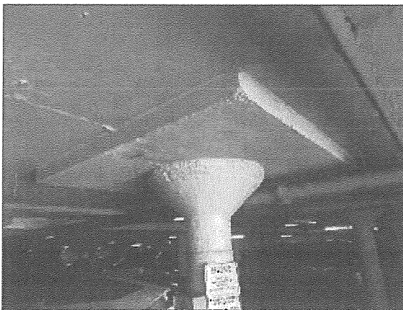
View of a typical column with a capital and drop panel supporting a reinforced suspended slab.
