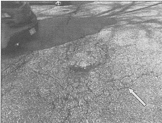
View of typical alligator cracking in the asphalt pavements located on the north portion of the Site.
