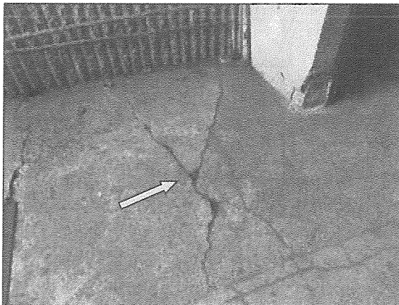
View of typical cracking in the cast-in-place concrete walkway noted adjacent to the loading area.
