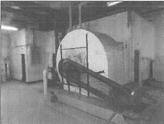
View of a typical central station built-up AHU located in the mechanical penthouse.
