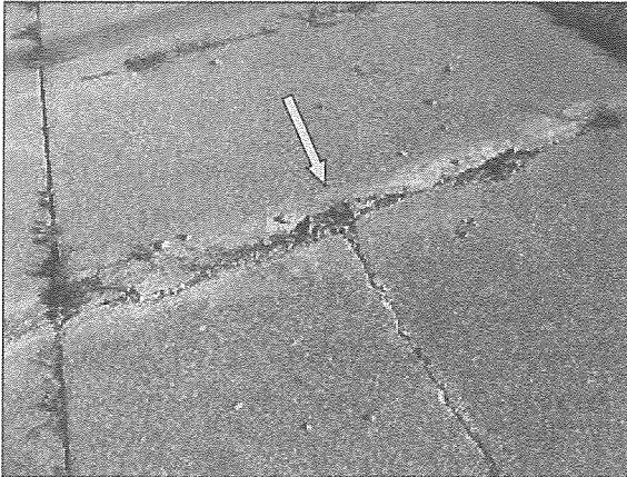
View of cracking in the cast-in-place concrete walkway noted adjacent to the south elevation.
