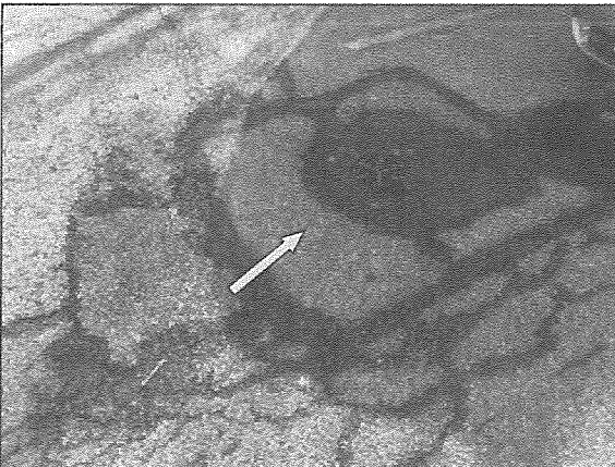
View of typical settled and deteriorated asphalt pavements around a drain in the podium deck noted on the east portion of the Site.
