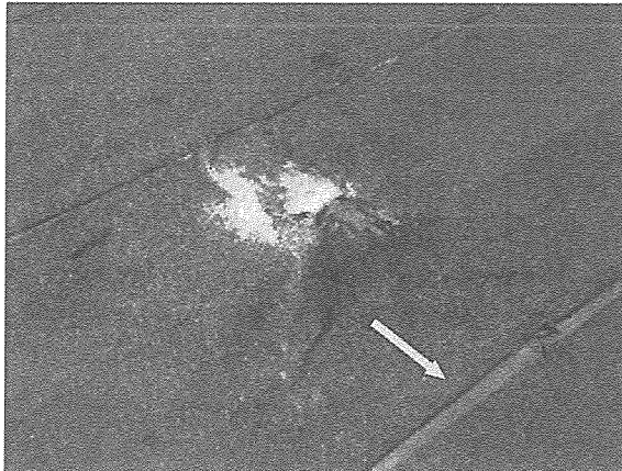
View of a deteriorated/failed seam in the modified bitumen membrane overlay noted atop the main roof level.
