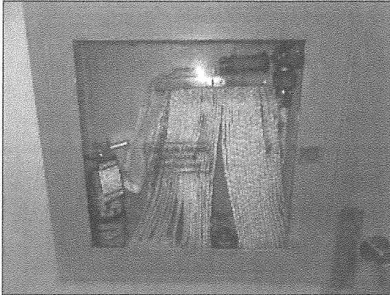
View of a typical fire hose cabinet complete with a chemically-charged ABC-class fire extinguisher.
