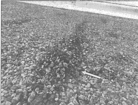
View of a typical blister in the BUR membrane.
