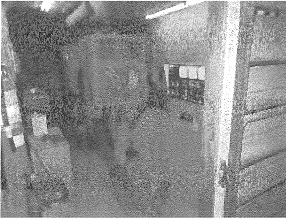
View of the diesel fire backup generator located in the UPG level generator room.
