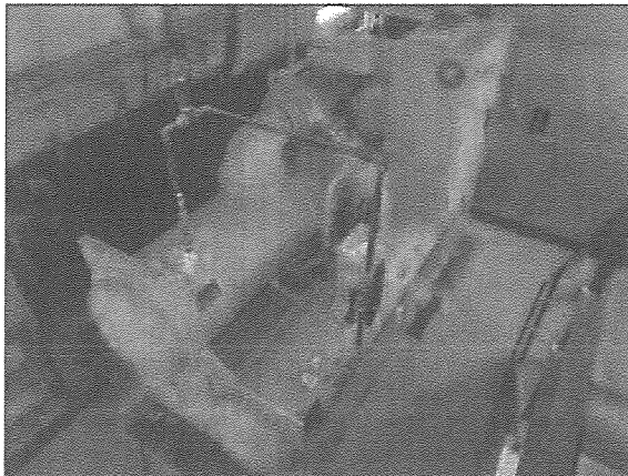
View of the chiller located in the mechanical penthouse.
