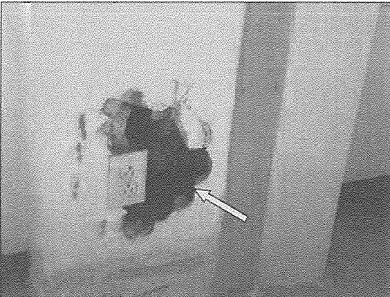
View of damaged gypsum wall board noted within a 2 nd floor vacant office space.
