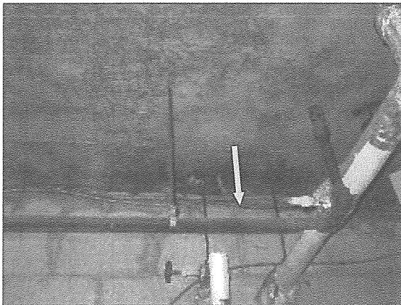
View of typical corroded sprinkler piping noted within the basement areas.
