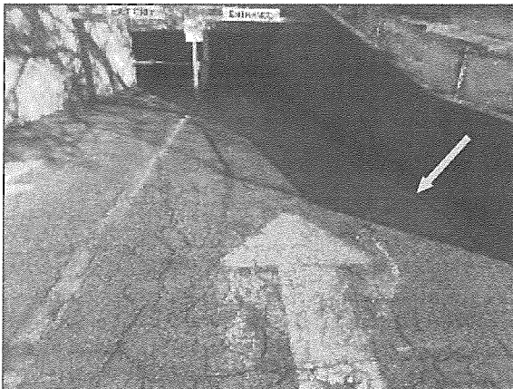
View of typical alligator cracking and deterioration in the asphalt paved UPG ramp located on the south portion of the Site.
