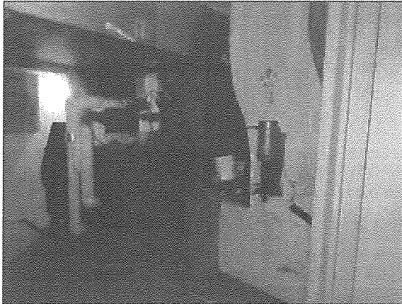
View of the AHU in the basement mechanical room.
