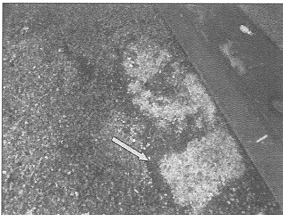
View of typical cement deposits in the BUR membrane.
