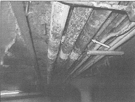
View of extensively corroded drainage piping noted within the UPG.
