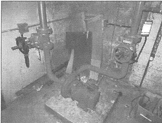
General view of the fire pump.
