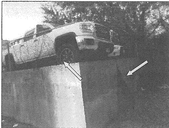
View of damaged chain link fencing noted on the northwest portion of the Site.
