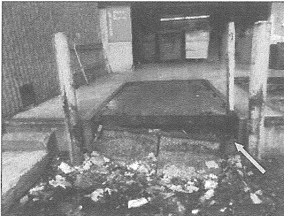
View of a damaged loading dock leveller noted in the loading area adjacent to the north elevation of the Site Building.
