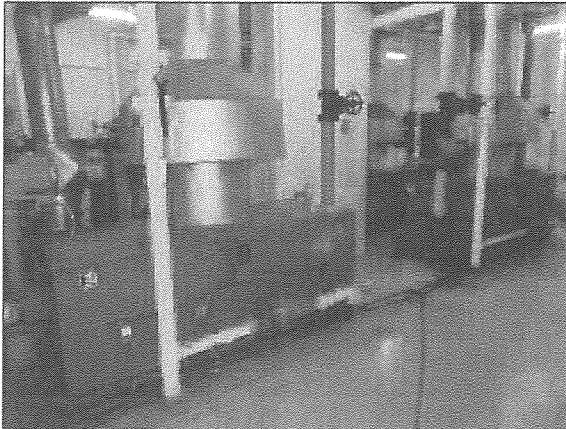
View of the natural gas-fired heating boilers located in the mechanical penthouse.
