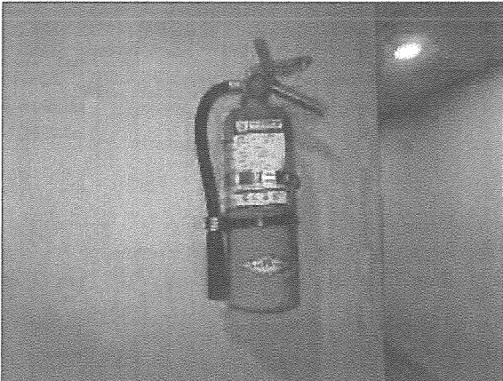
View of a typical wall mounted chemically-charged ABC-class fire extinguisher.
