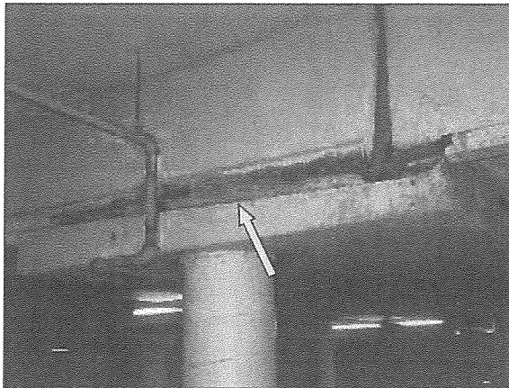
View of an extensively corroded metal trough noted within the UPG.
