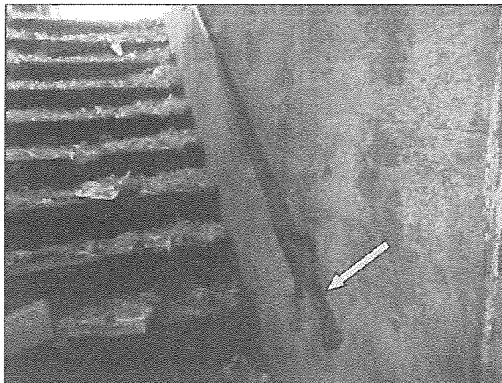
View of an extensively corroded steel handrail noted in the west emergency exit stairwell.
