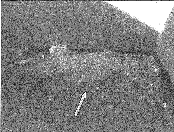
View of typical debris noted atop the BUR system within the vicinity of the cooling tower.
